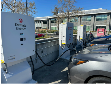
Figure 1: EVs and bidirectional chargers at the research site.
